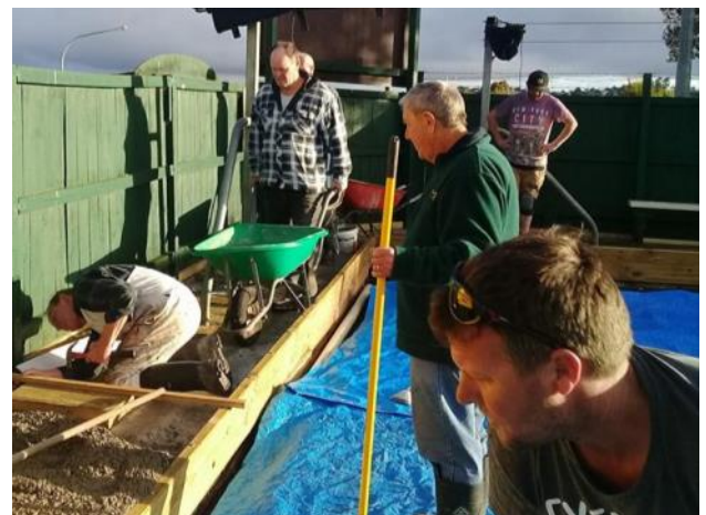
It was all go Saturday morning as the concrete went down around the bottom green, a job well done.
